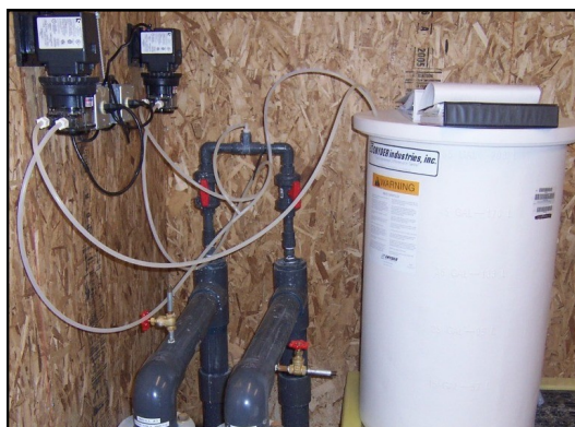
Chlorine injection system. Photo by Paul Kim.
