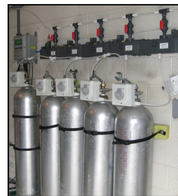
Gas chlorine cylinders. Photo by Serenity Valdez.
